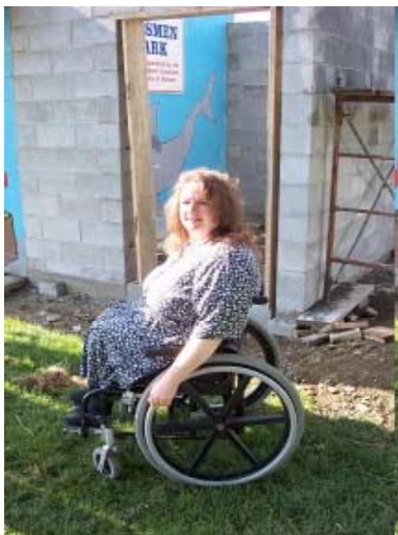
Christine Paisley from the Cowichan Valley Disability Resource Centre conducts on-site of handicap washroom under construction at Kinsmen Park
